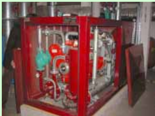
The installed CHP plant
