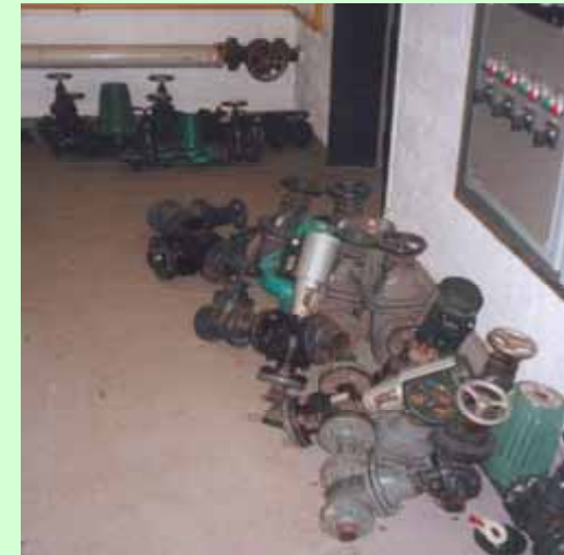
Old pumps - not needed anymore
